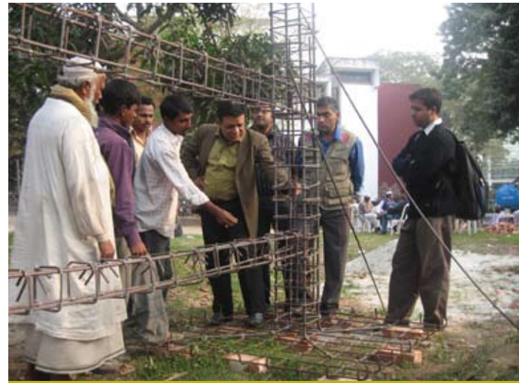
Briefing about the earthquake resistant technique during the mason training in Bangladesh
